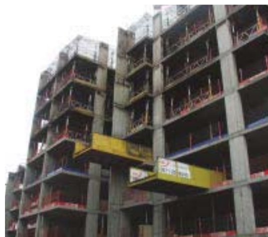
Figure 2: The concrete frame of a ten-storey building that was fire-damaged during construction.
