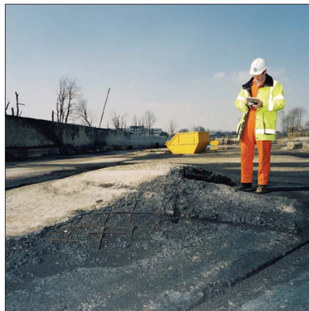
Figure 7. Fire-damaged reinforced concrete floor at tank 12 bund
