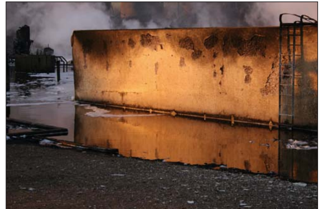
Figure 9. Leaking tie-bar holes in tank 12 bund (at lower part of bund)
