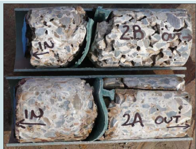
Core 2B: taken through the wall of bund E, showing very little heating damage to the concrete and no evidence of damage to the polyvinyl chloride water stop.
