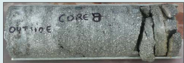
Core 8: taken through a repaired area of main bund showing laminar striations in the outer 50 mm of the wall, but generally very good performance for the sprayed concrete material.
