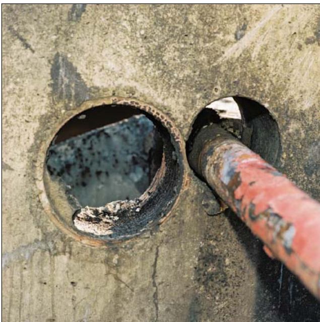
Figure 8. Bund pipe penetrations (lacking puddle flanges)
