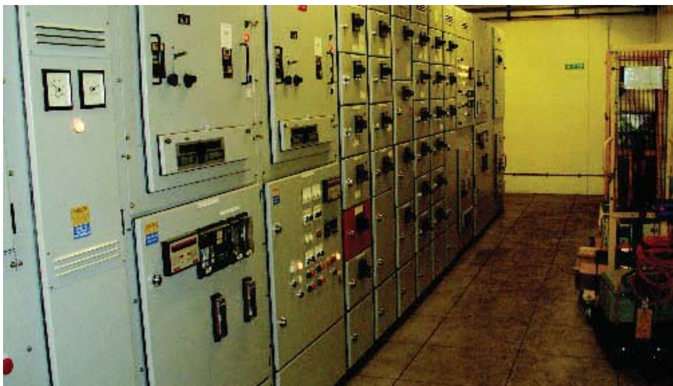
Control centre at Medway Tunnel
