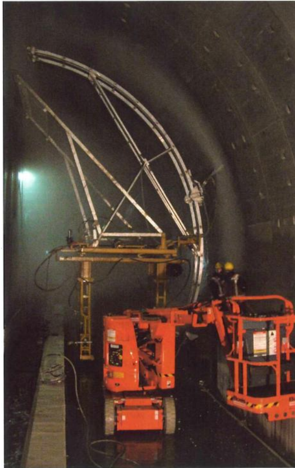
Figure 4: Application of cementitious fire protection lining to the Groene Hart Tunnel (Gijsbers et al, 2006)
