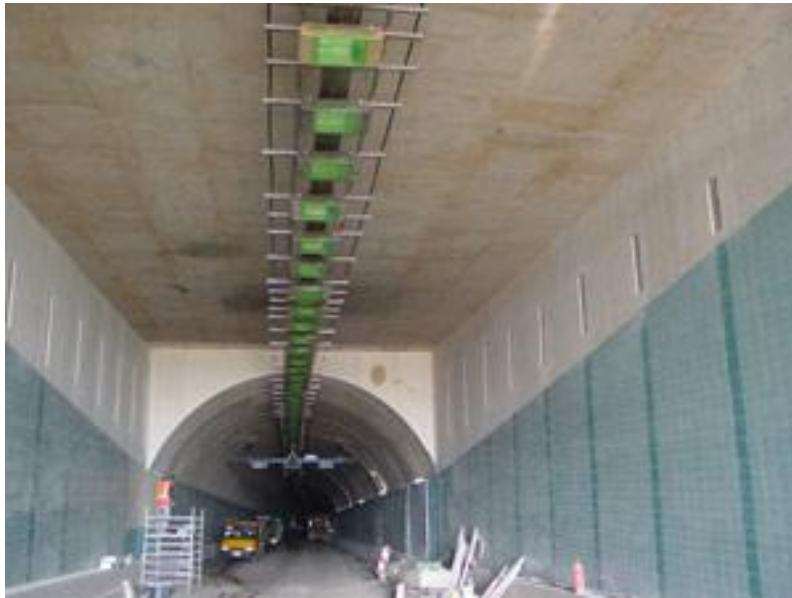
Figure 3: Westerschelde Tunnel, Netherlands (showing fire protection boards on ceiling and the upper part of the walls).
