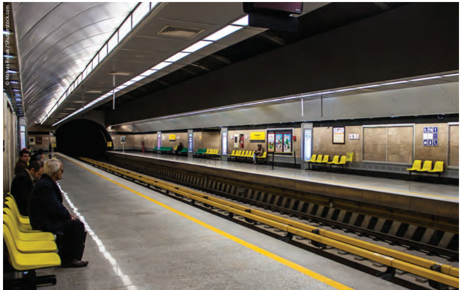
Air-conditioned air flows into the Tehran Metro tunnels and a reduction in the tunnel temperatures can thus be achieved
