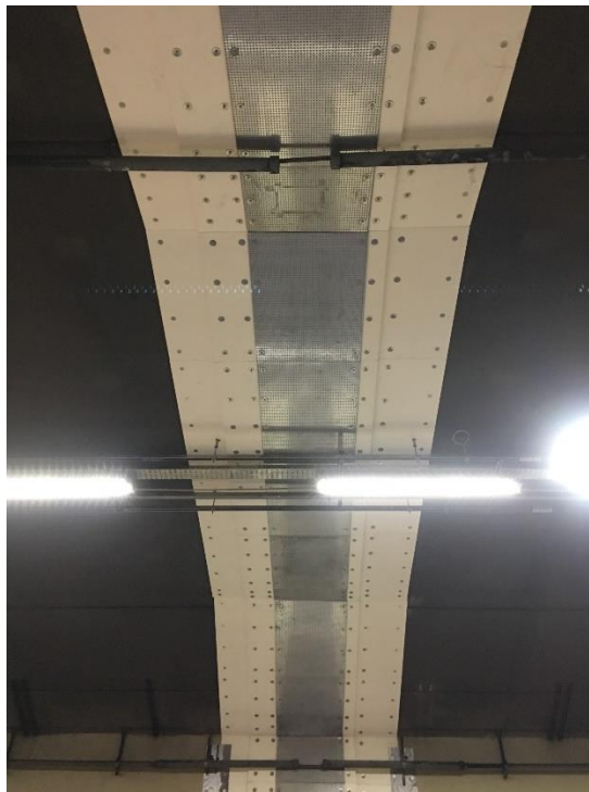
Figure 15: Passive fire protection boards installed on tunnel soffit
