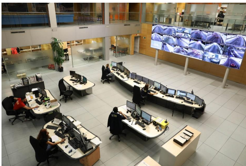
Figure 3: Main Control Centre.
