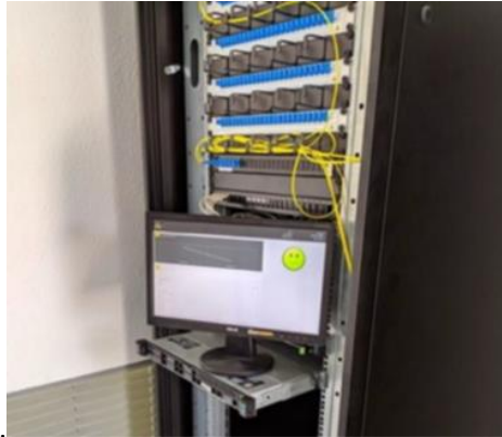
Figure 7 - An example of SCADRA installation
