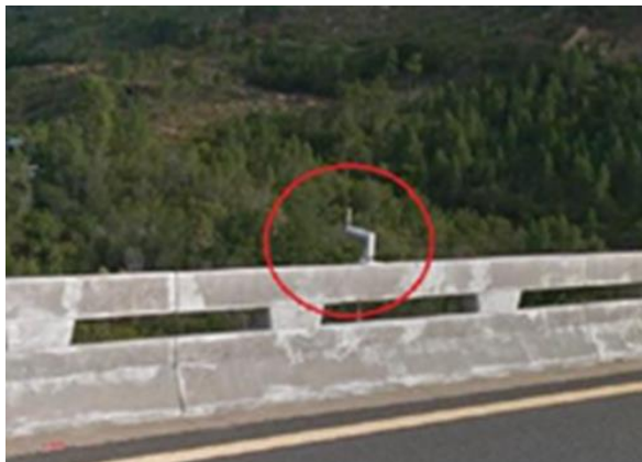
Figure 2 - Weather station on the Hugo River Viaduct
