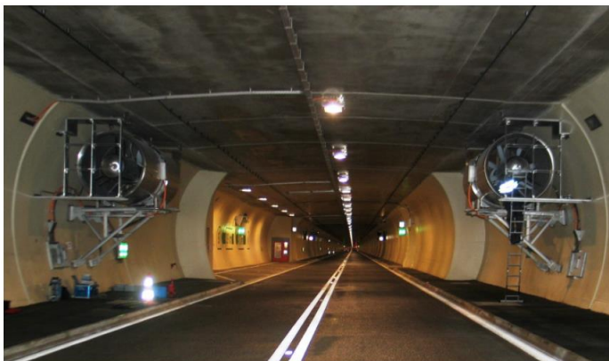
Figure 4: Bosruck tunnel jet fans (Beyer et al., 2016)
